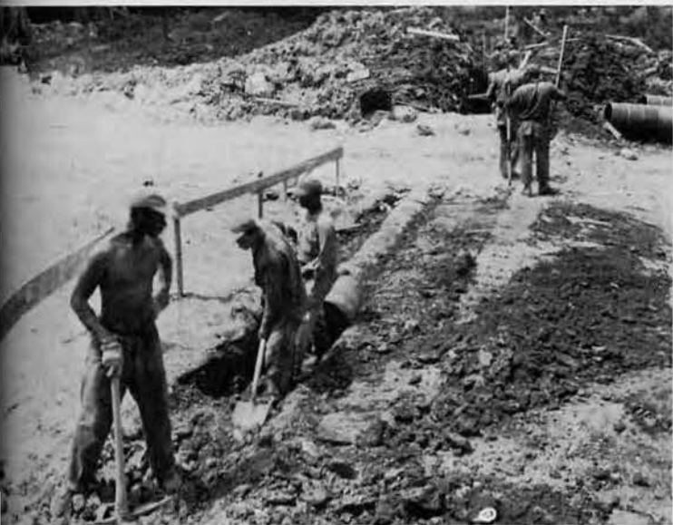
Culvert made from oil drums being installed beneath Route #8 which drains 34th Transportation area and main road.
