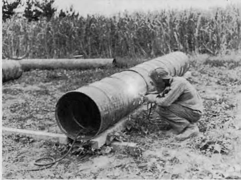
The old adage "Necessity is the Mother of Invention", or the Seabees motto, "If you haven't got one, make one", is shown in this picture. A drum of gasoline was shipped from the States, contents used in a truck or tractor—now the empties are welded together for very efficient culverts.
