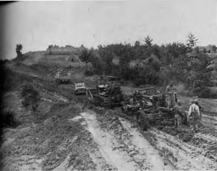
Highway #8 at outskirts of 34th Camp. Even at this stage, there is a great improvement over the muddy, deep rutted trail we found.
