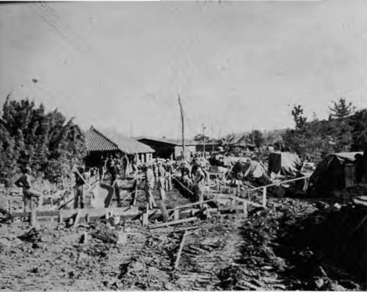
Forms being set on 1½ Quonset Huts for Chiefs' Mess. With 52 Chiefs in the Battalion at this time, ample room will be assured with this size building.
